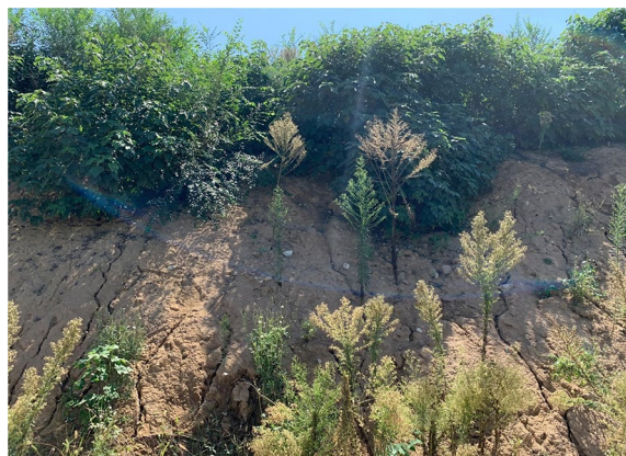
Fig. 11 Cracks in the sections of the wall directly exposed to the external environment
