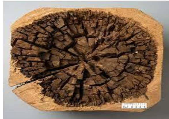
Plate 7B: Decay fungal growth on wooden
