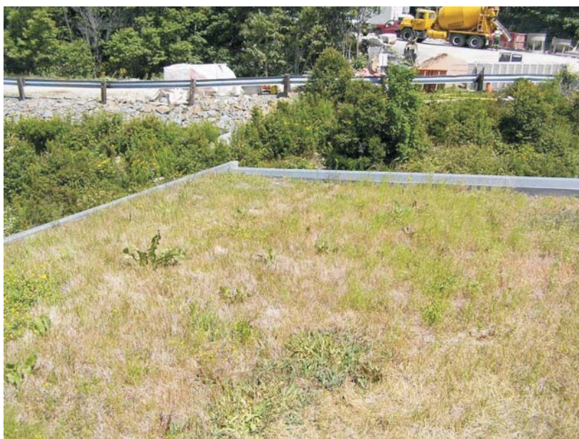
An extensive green roof. Shallow soil requires plant species adapted to extremes of moisture and temperature.
