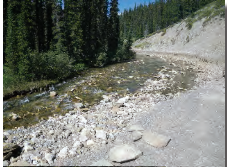
Road washout south of the Cardinal Divide in summer 2013. Photo S. Pittman
