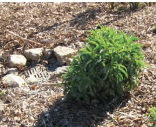
A dry well inlet in Old Marengo Park was discovered after a pile of mulch that had been covering it was removed. The underground dry well detains and infiltrates stormwater that flows across the site. Photograph by Ellen Mackey.
