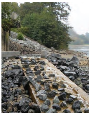
Figure 2: An example of human-engineered stream flow – ramp with baffles (UK)
