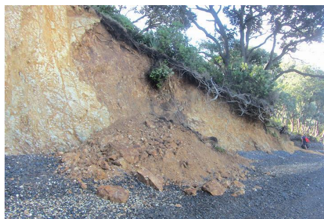
Fig. 3. Eroding coastal cliff face at Otata beach by the bach after a severe storm. Photo: 11 Oct 2016. If not otherwise stated, all photographs are by the author.
