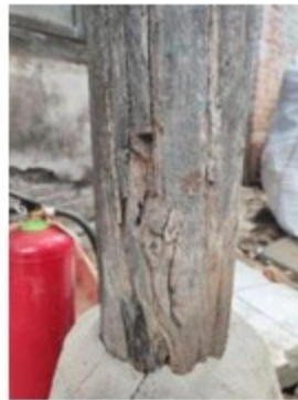
(e) Decay of column bases
