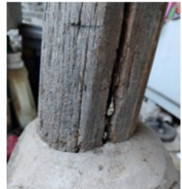
(f) Decay of column bases
