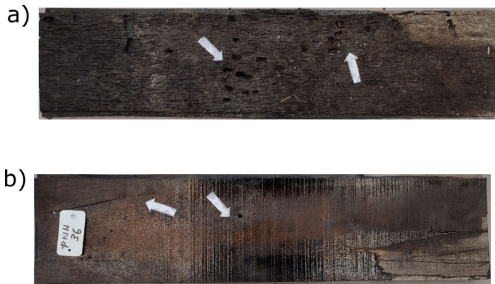
Fig. 2 Detrioration on water side (a) and earth side (b), with arrows highlighting the holes due to marine borer attack
