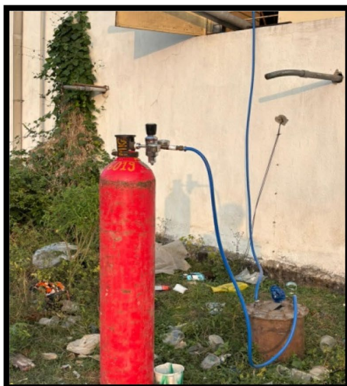
Hydrogen Gas supply
